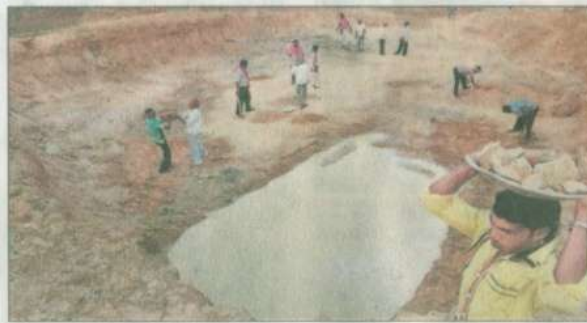
Villagers in Bengal's Purulia district dig a large catchment area for rainwater harvesting.
