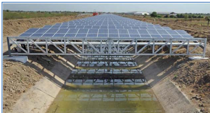
Canal Top Solar PH over Narmada Canal near Vadodara
